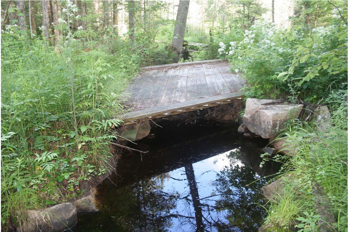
Photo # 7 description: B&M Bridge 222, Bethlehem. 3350' south of Trudeau Rd. crossing. Wood stringer (recently rebuilt) on rebuilt split fieldstone abutments, ~8' span. nd.
