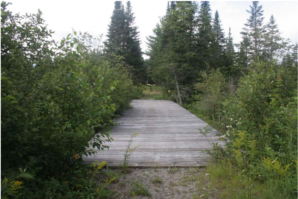
Photo # 9 description: Beaver Brook Bridge, Profile Recreational Trail, Bethlehem. Newly constructed trail bridge on new stone abutments; probably utilized some split fieldstone from previous bridge.
