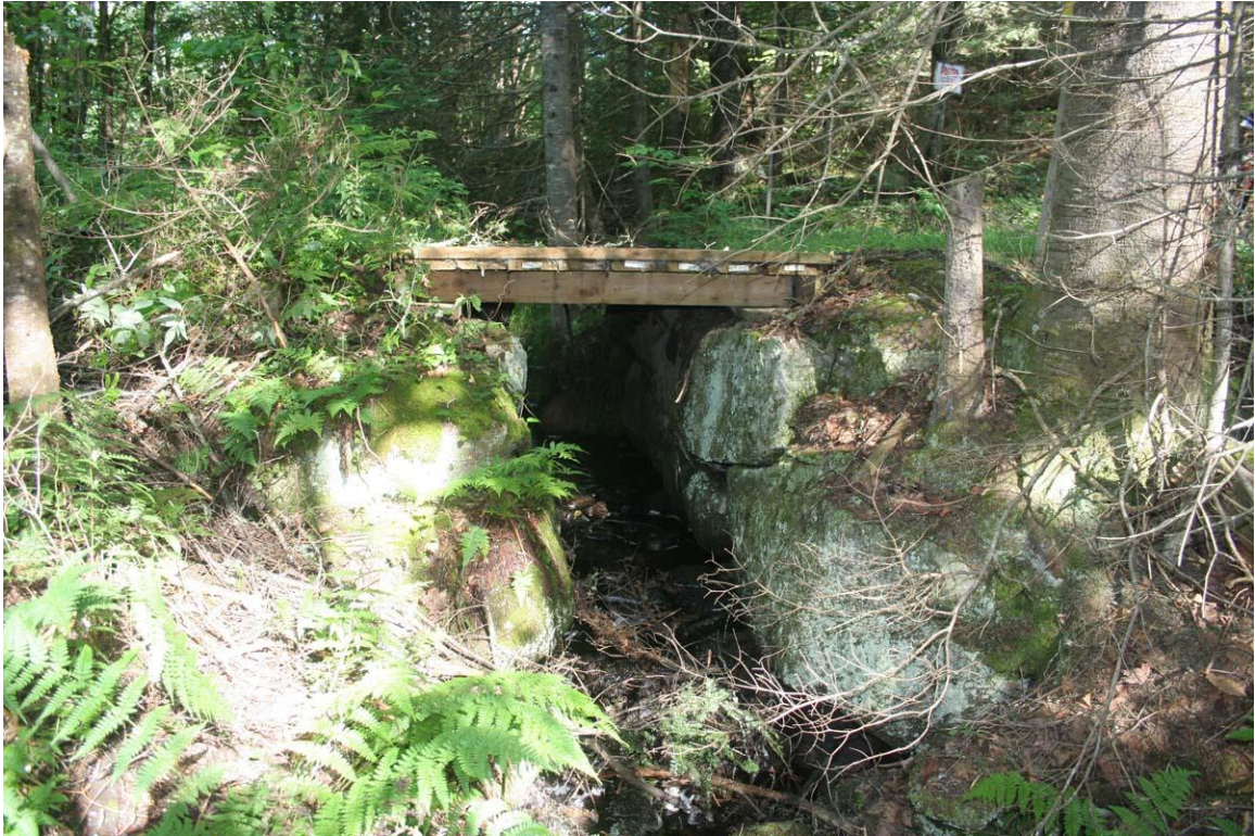
Photo # 5 description: B&M Bridge 222b, Bethlehem. 2750' south of Trudeau Rd. crossing. Wood stringer (recently rebuilt) on split fieldstone abutments, ~4' span. nd.
