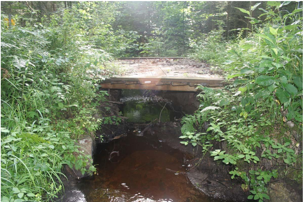
Photo # 6 description: B&M Bridge 222c, Bethlehem. 3100' south of Trudeau Rd. crossing. Wood stringer (recently rebuilt) on split fieldstone abutments, ~5' span. nd.
